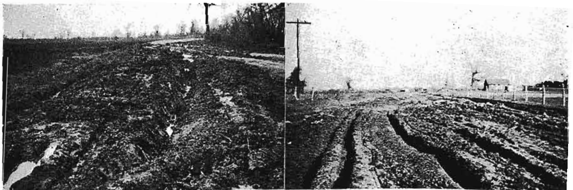
The Result of Alternate Freezing and Thawing of Gravel Roads
